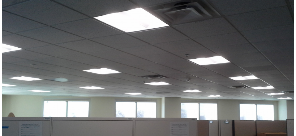
In a lighting upgrade of the New Carrollton Federal Building in Lanham, Maryland, the General Services Administration cut energy use by 82% and trimmed an annual lighting bill from $291,000 to $53,500 by replacing 11,800 fluorescent troffers with LED fixtures and controls. Photo source: GSA.
